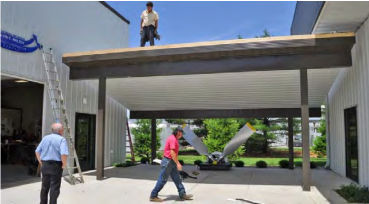
The canopy joining the new workshop to the main museum building was completed in June.
